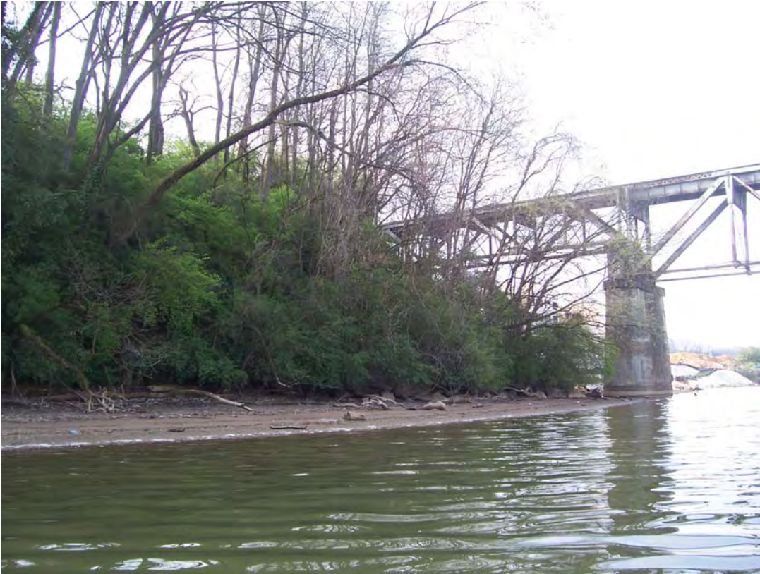
Photograph #BT-47. View to southeast of shoal area in Project 6 and Norfolk Southern Railroad Bridge.
