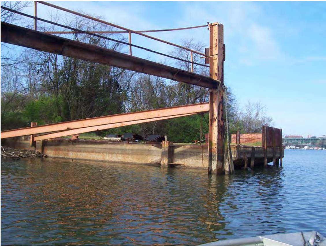
Photograph #BT-15. View to southwest of metal barge pier and floating dock on Project 10 site. Shoal area continues under floating dock.
