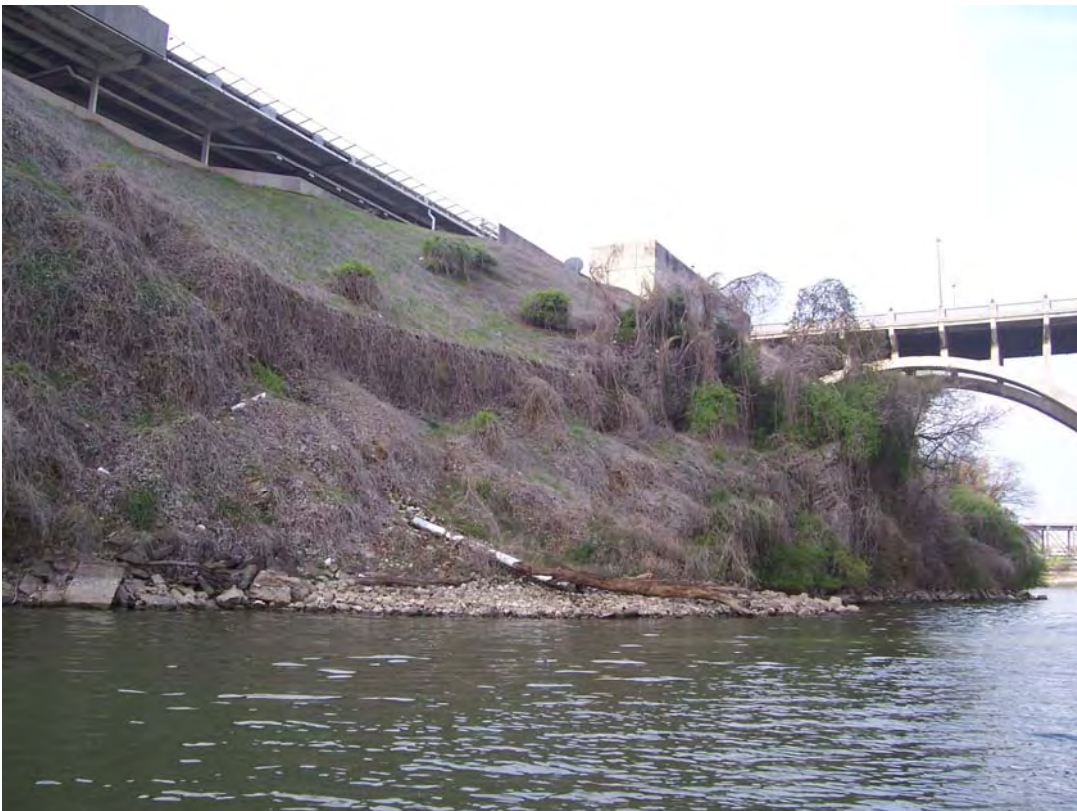
Photograph #BT-36. View to southwest towards Henley Street Bridge. Bluff and shoals area.
