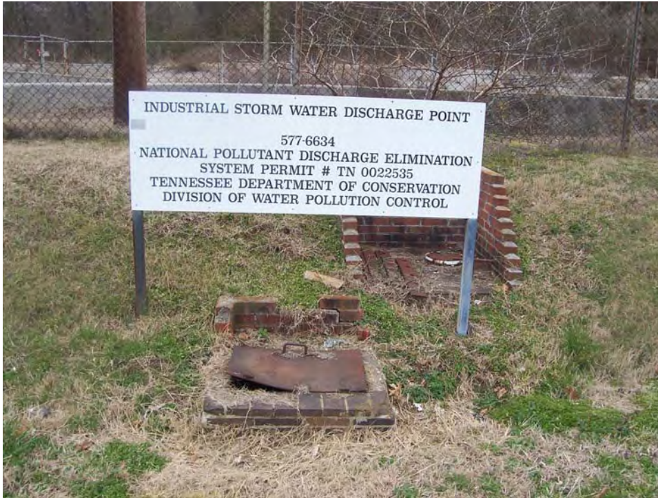
Photograph 11-3. View to southwest of NPDES permitted outfall at former Transmontaigne tank farm site on Island Home Avenue.
