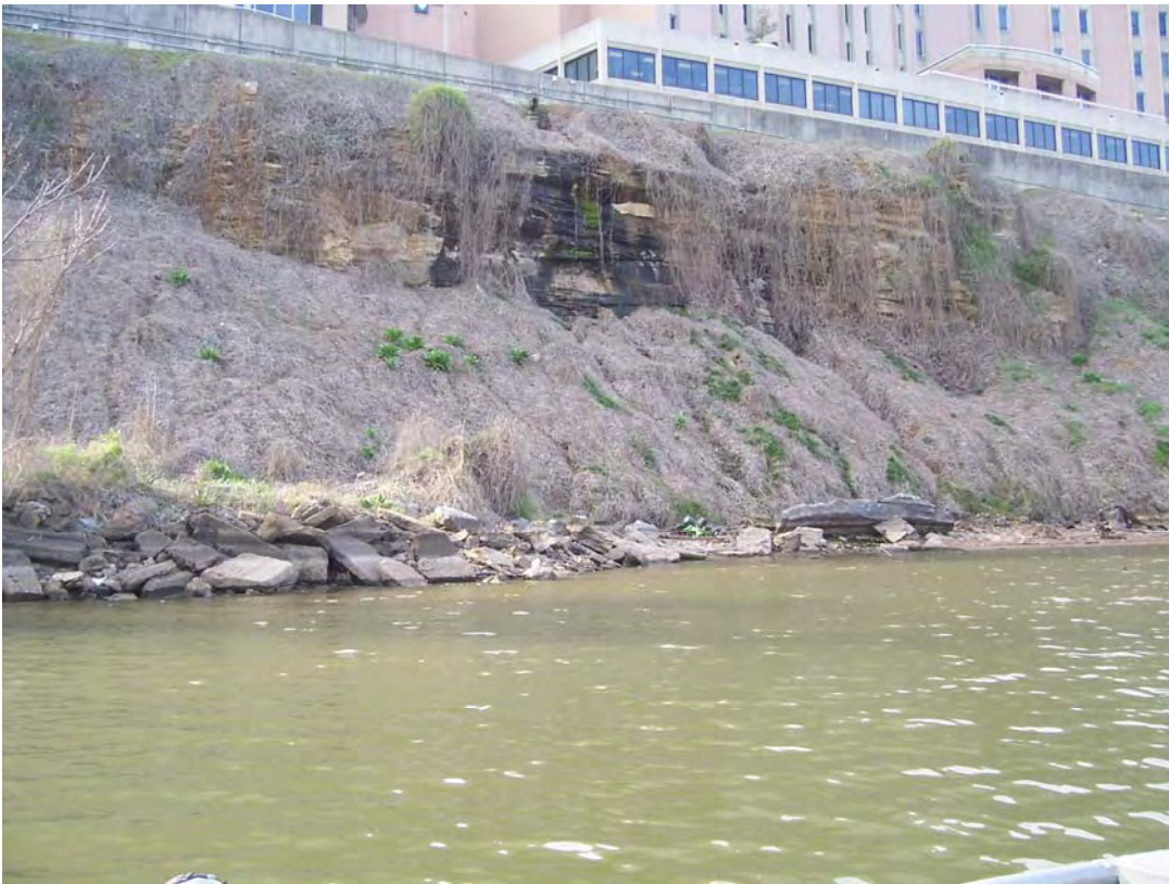
Photograph #BT-31. View to southwest. General stormwater drainage from Baptist Hospital onto bluffs. Continuous drainage has created habitat for mosses to grow on the limestone outcropping (area of dark colored rocks). Shoal area evident in foreground of photograph.
