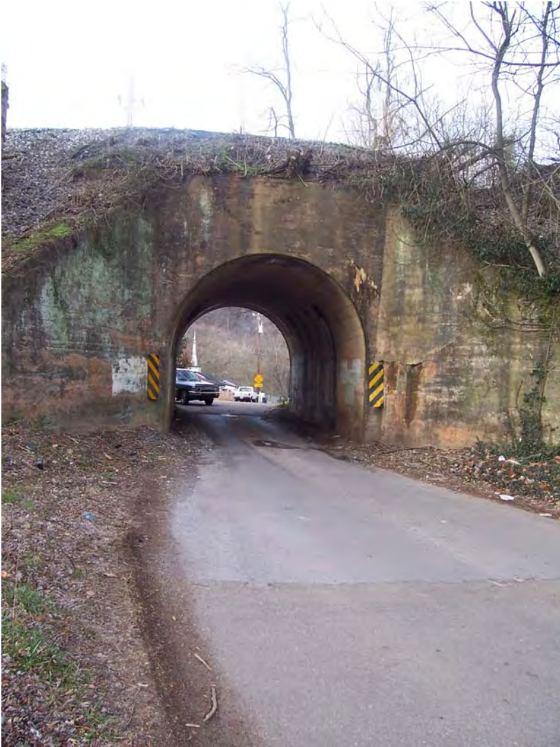
Photograph 1-9. View to west. East side of underpass at Scottish Pike/Cherokee Trail intersection.
