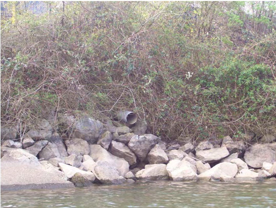
Photograph #BT-20. View to south of outfall for general site stormwater drainage from the Project 9 site. Outfall located east of metal barge piers and near the eastern portion of the large building on the Project 9 site.
