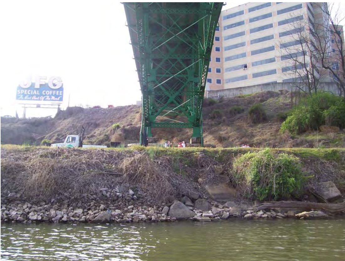
Photograph #BT-28. View to south underneath Gay Street Bridge of Project 7 site.
