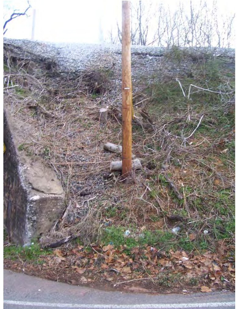
Photograph 1-4. View to east. West side of railroad at Scottish Pike/Cherokee Trail intersection
