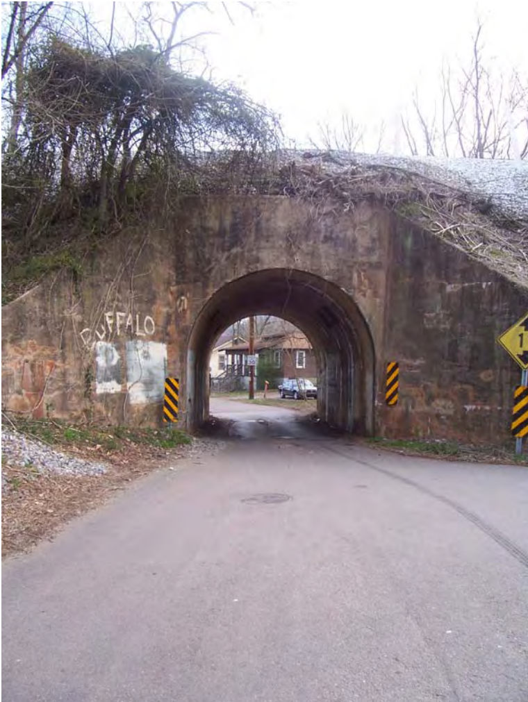
Photograph 1-3. View to east. West side of underpass at Scottish Pike/Cherokee Trail intersection.
