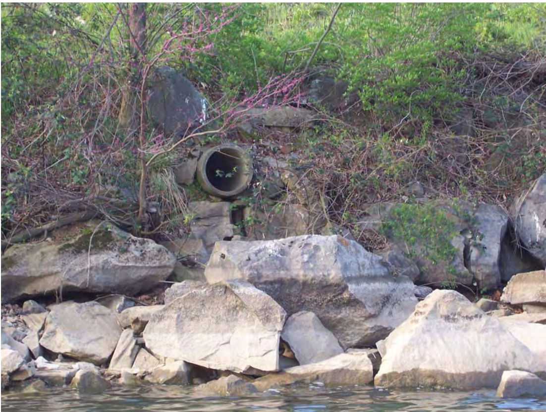
Photograph #BT-4. Outfall for Industrial Stormwater NPDES permit TN0022535 from former TransMontaigne Fuel Tank Farm property on Island Home Avenue. Outfall located in western end of Project 11 in rip rap area.
