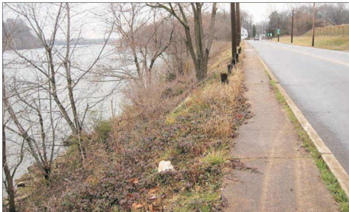
11B. Steep Embankment, West Portion of Baker Creek Landing Area
