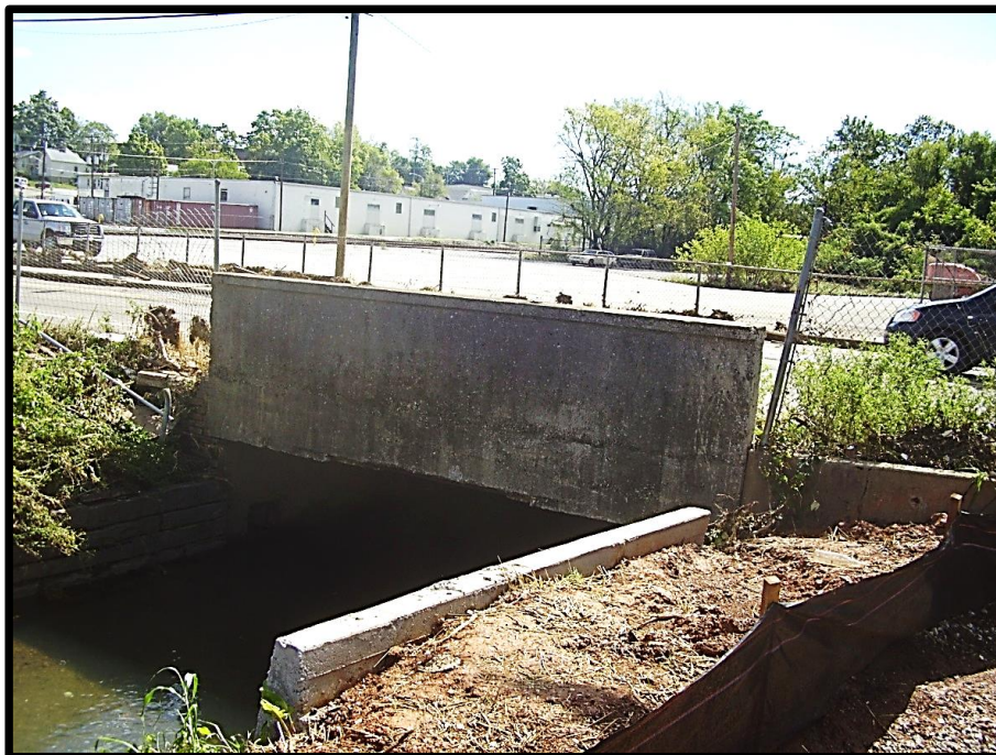
Photograph 16: View to the southeast of the condition of Second Creek entering the subject area through a box culvert underneath Baxter Avenue.
