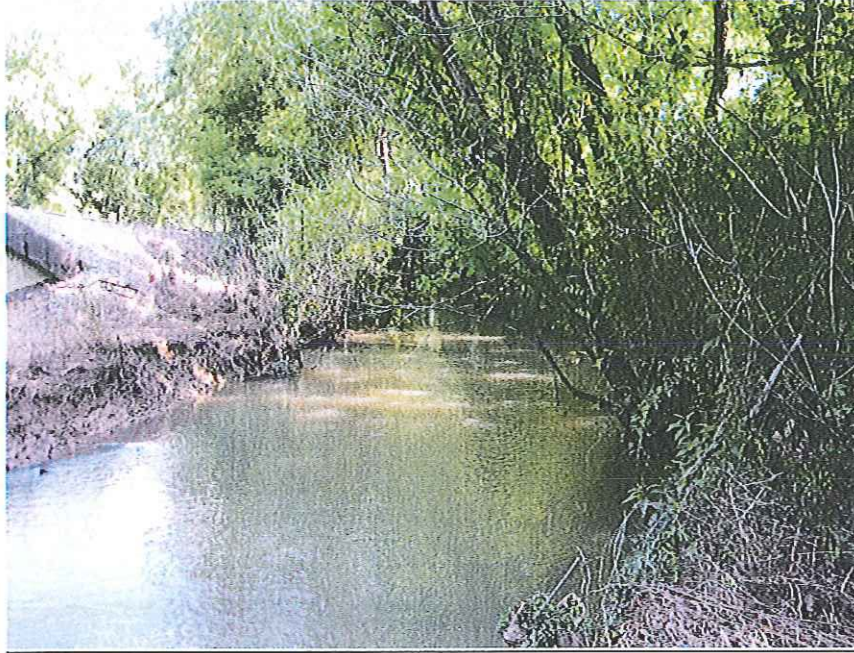
Photo 1. Upper site showing bank failure.
