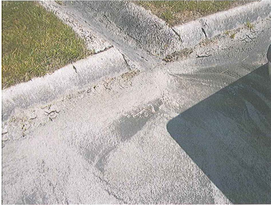
Photo 16. Evidence of sediment entering First Creek from a parking lot.
