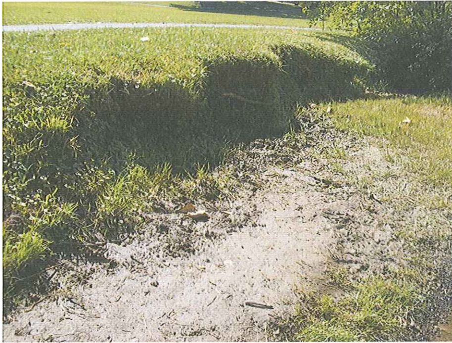
Photo 7. Bank failure located along the walking path.
