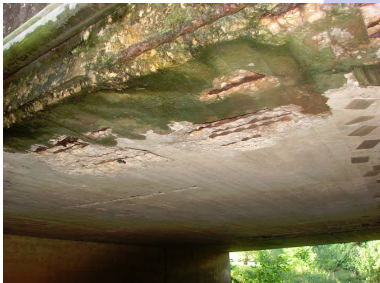
Spalling with Exposed Rebar
