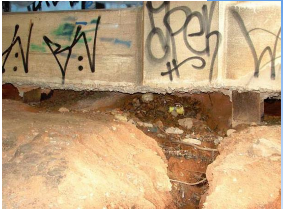
Exposed Piling Beneath the Ed Shouse Drive Bridge
